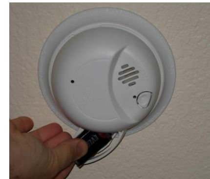
Typical Battery Replacement
