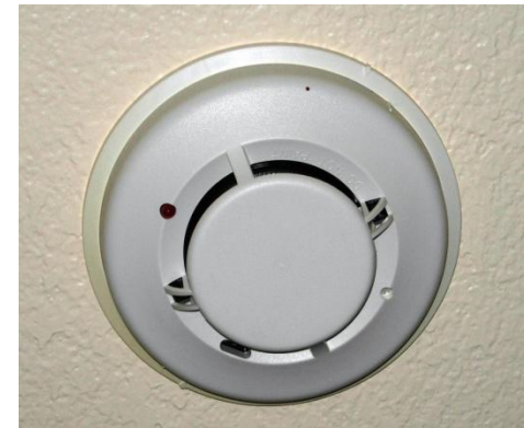
Smoke Sensor Wired to Security Alarm
