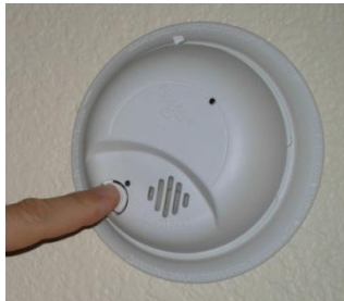
Testing the Smoke Alarm
